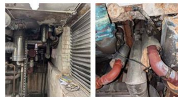
Visible damp and water ingress in basement plant / boiler room. Areas of concrete were spalled and some visible steel members with surface rusting.
