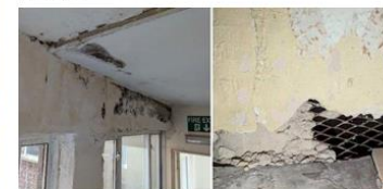
Damp and mould present above some windows at upper levels. Some partition walls and finishes are in poor condition with visible holes
