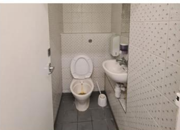
Typical shared WC
