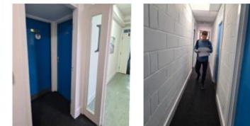
Narrow corridors to bedrooms and some rooms directly accessed from core lobby which could potentially pose fire and safety risk hazard
